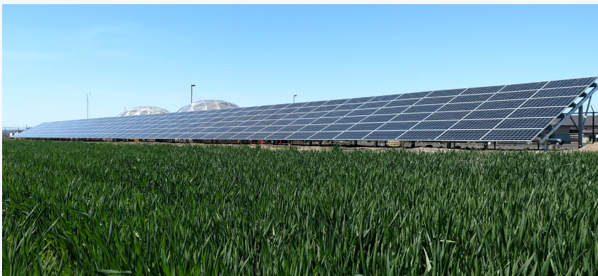
The Ántukš-Tiínqapapt or “sun trap” solar array recently installed by the Confederated Tribes of the Umatilla Indian Reservation in Oregon. Source: DOE.
